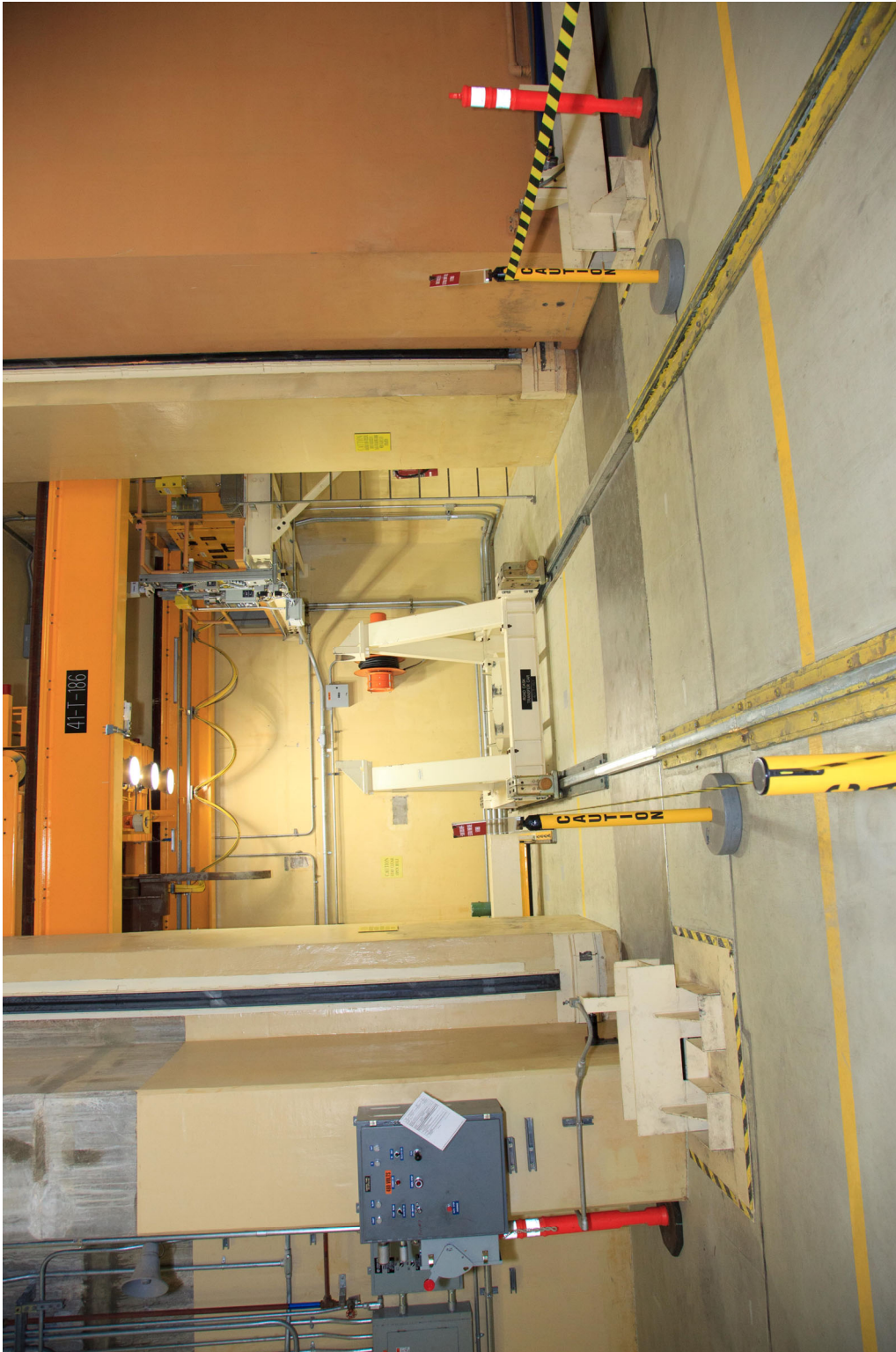
Figure B4-8 Cask Unloading Room and Bridge Crane
