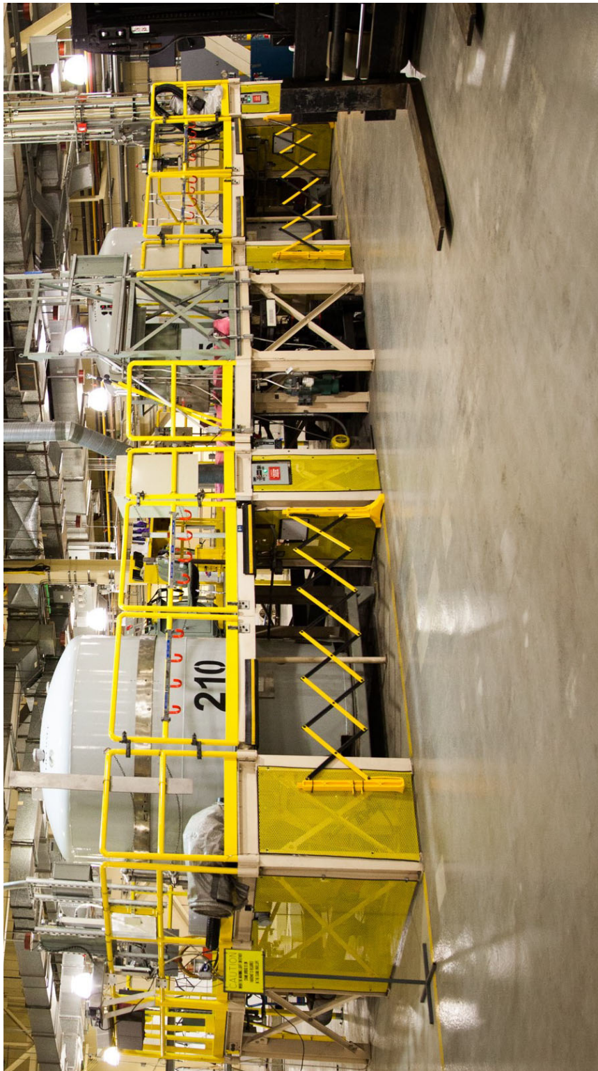
Figure B4-4 TRUDOCK (East) in CH Bay of the Waste Handling Building
