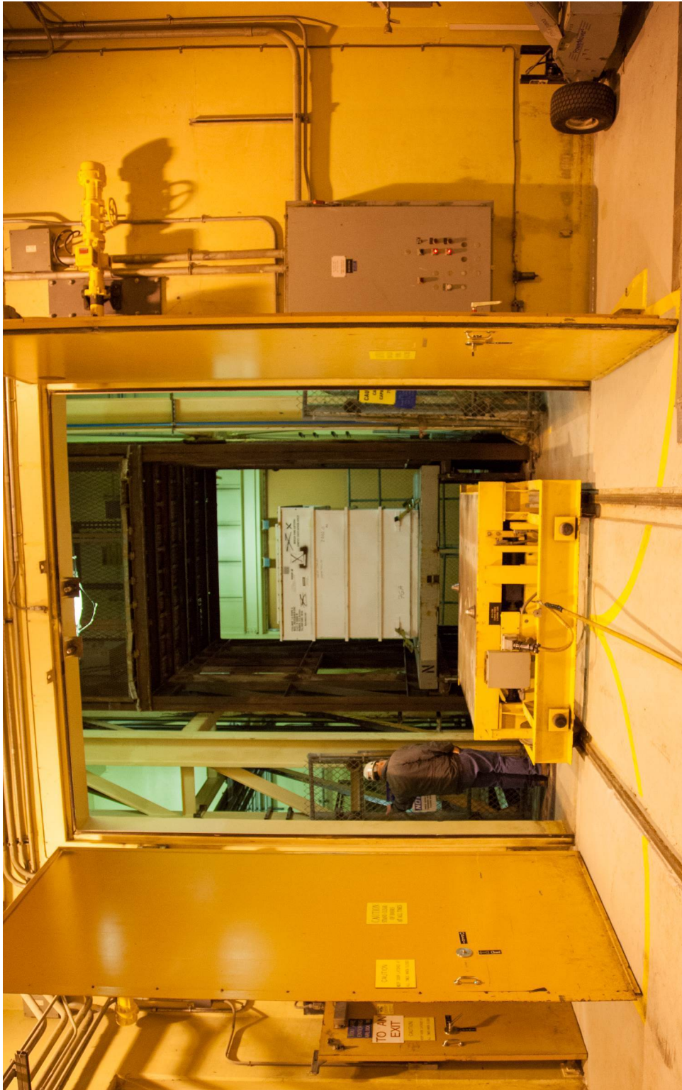
Figure B4-6 Waste Shaft Conveyance - Loading Facility Pallet with CH Waste, Waste Handling Building
